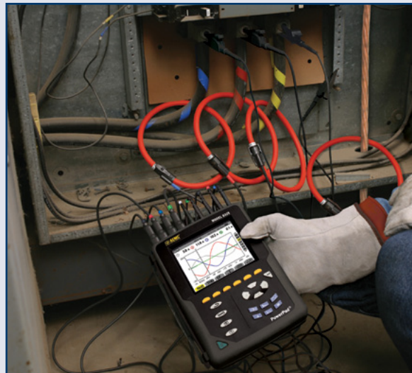
Power quality analysis on a three-phase panel using the AmpFlex ® flexible current probes.
