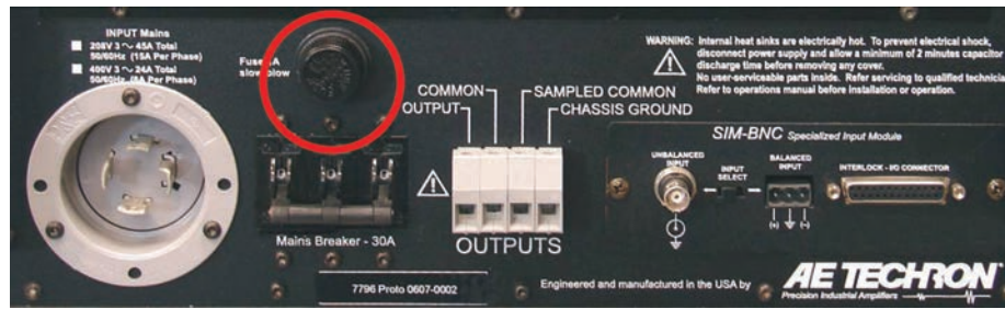
Figure 8.3 – Fuse F1 Location
