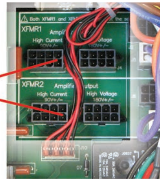
Figure 5.10 – Location of Amplifier High-Voltage Transformer Sockets
