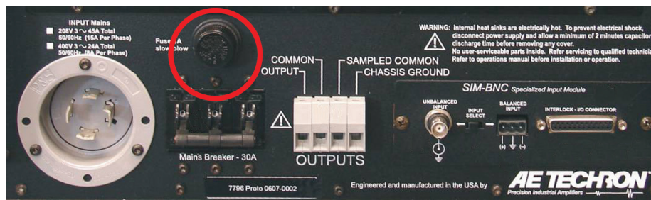
Figure 7.3 – Fuse F1 Location
