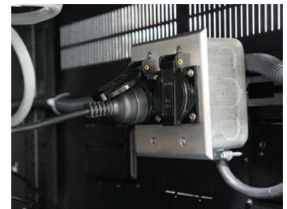
Figure 6.3 230V Auxiliary Outlets
