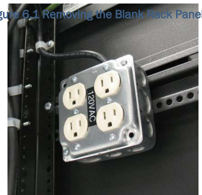
Figure 6.2 120V Auxiliary Outlets
