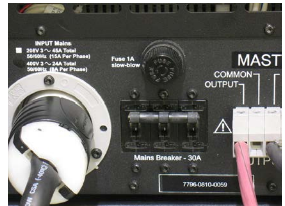
Figure 8.1 Back-Panel Circuit Breakers and Fuse F1 Location
